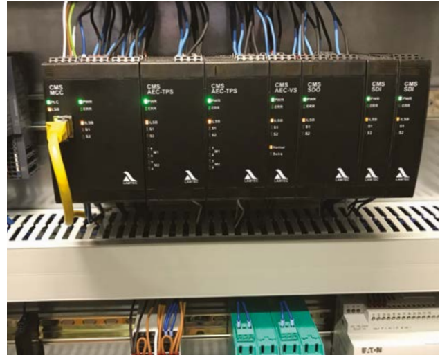
CMS modules installed in the control cabinet.
